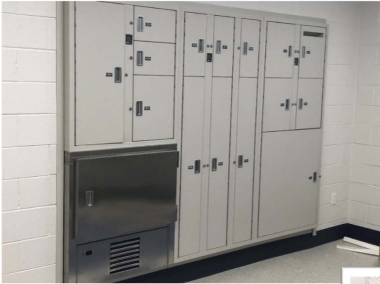
EVIDENCE TRANSFER LOCKERS
